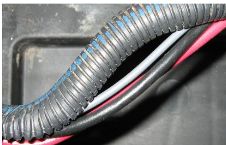
Figure 3: Receptacle Wires Exposed
